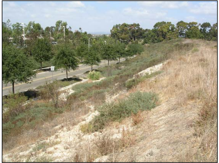
View north, looking at slope area to be graded between Innovation and Academy Way
