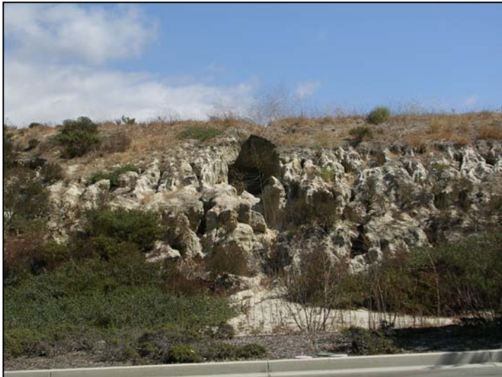
View of highly eroded slope within proposed grading limits
