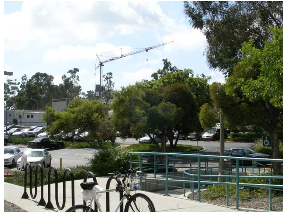
View west, from western edge of site, across Parking Lot 7, toward Central Plant.
